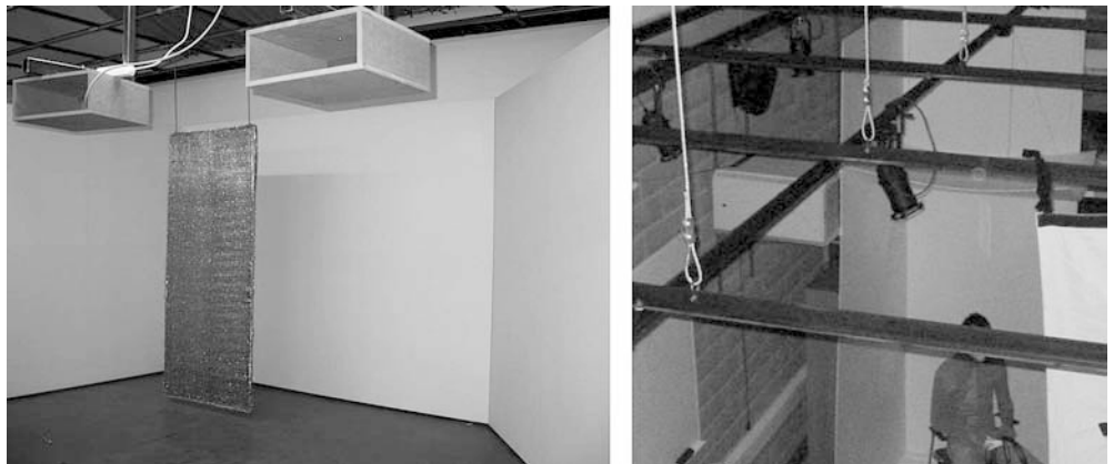
Fig. 5 Physical infrastructure for projection spaces
